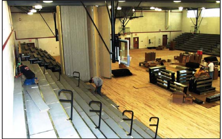
Workers install bleachers in the 1000-seat Mary Ellen Henderson Middle School Gym, which will be able to host regional tournaments.
